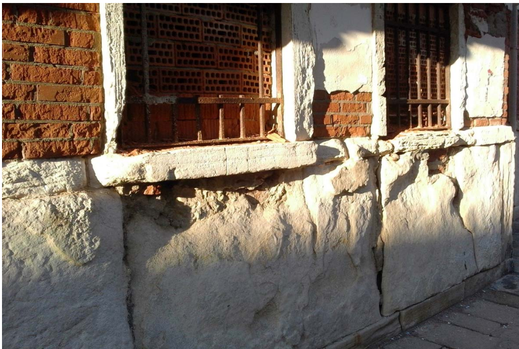
Palazzo Minotto, Fondamenta Briati (Orsoduro 2365-2371A): property of the Comune, closed and with bricked windows, abandoned and out of use since years, with important defects due to humidity (exterior and interior). (Bernhard Furrer, October 2015)
